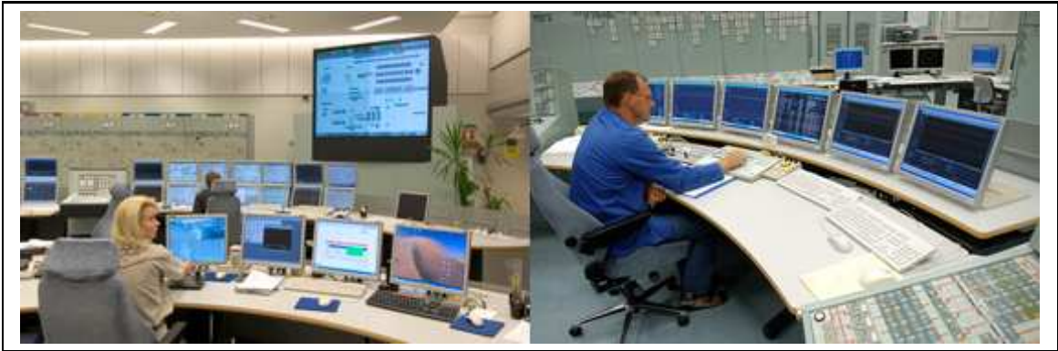
Figure 5.2: Pictures of Teollisuuden Voima (TVO) nuclear power plant process operator room.
