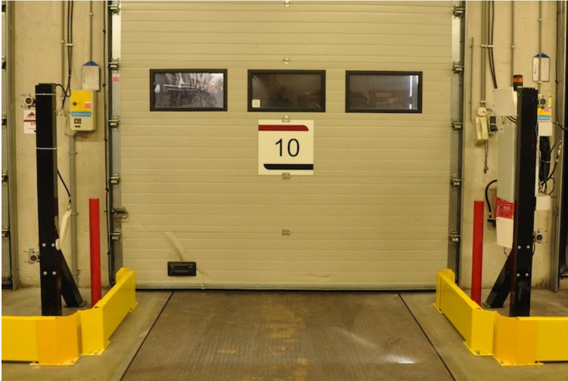
Figure 8: RFID Gate at docking door.
