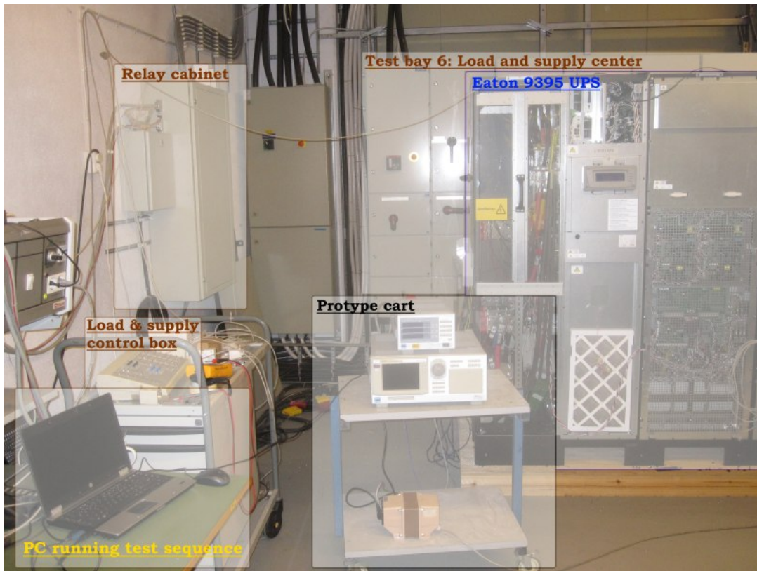
Figure 16: Efficiency test installation for the Eaton 9395 UPS.
