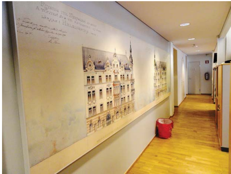
(a) Absorptive wall panel installed on the corridor wall.
