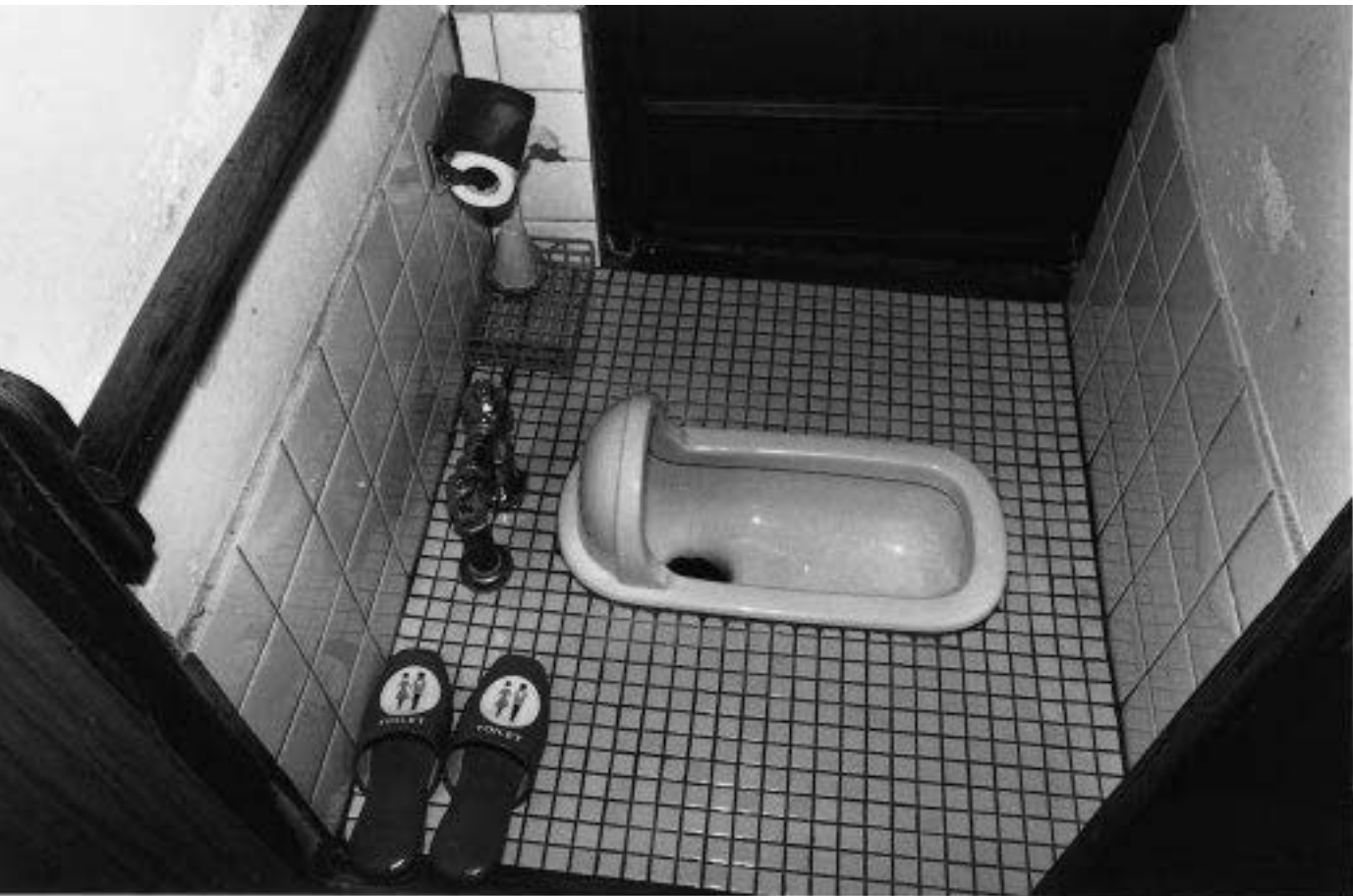
FIG.86 OTEARAI. THE JAPANESE STYLE TOILET. THE SUGIURA HOUSE. RS.
