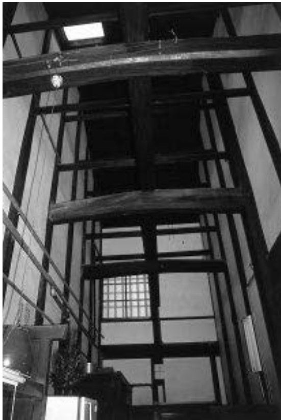
FIG.76 INTERIOR OF THE NAKAE I HOUSE. VIEW FROM THE EARTH FLOOR AREA, TŌRINIWA. RS.
