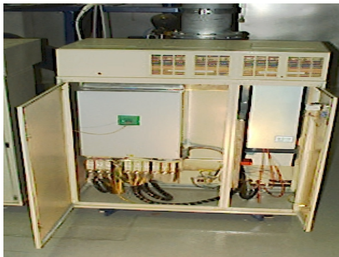
Figure 4. Six 250 kW, 32000 1/min. turbocompressors running in a water treatment plant in Finland. At the right-hand side the frequency converter and the AMB control electronics.
