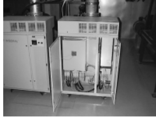
(b) The electric units, the frequency converter and AMB-controller
