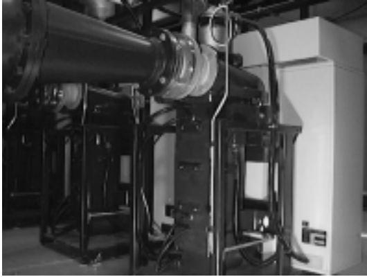
(a) Several high-speed turbo compressors in parallel operation
