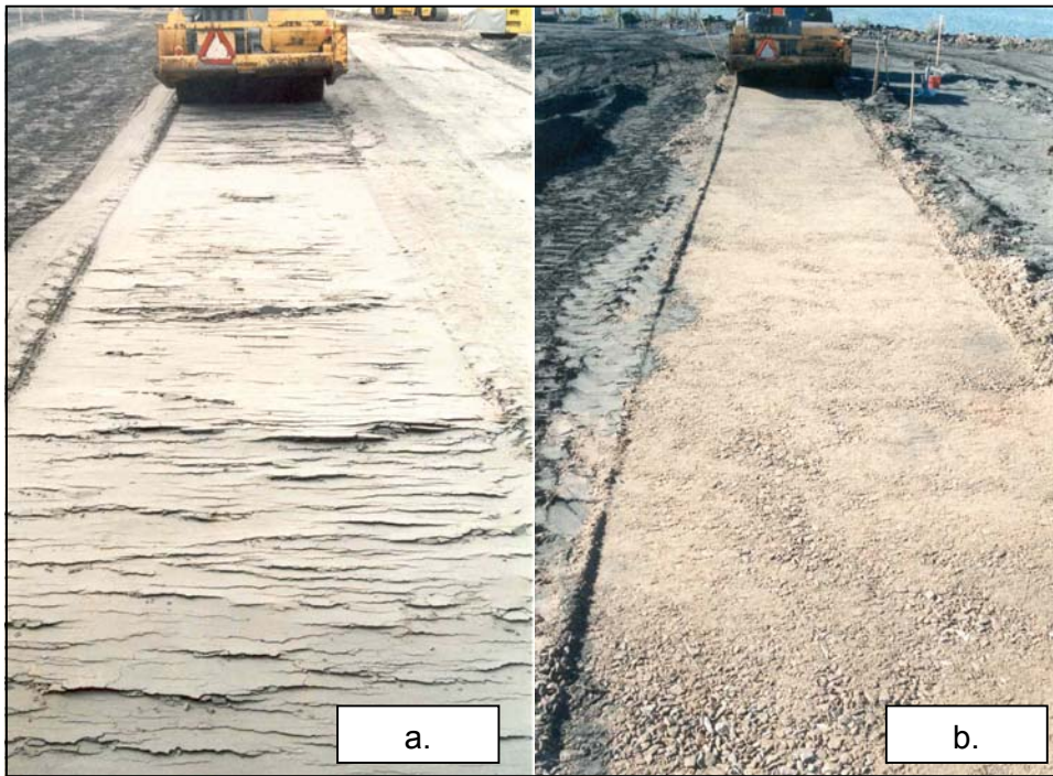
Figure 5-12: Testing of the FA compacting methods [6]; a) A Smooth Drum Vibratory Soil Compactor is compacting deep but leaving a scalelike surface which b) can be compacted through a thin course of crushed stone.
