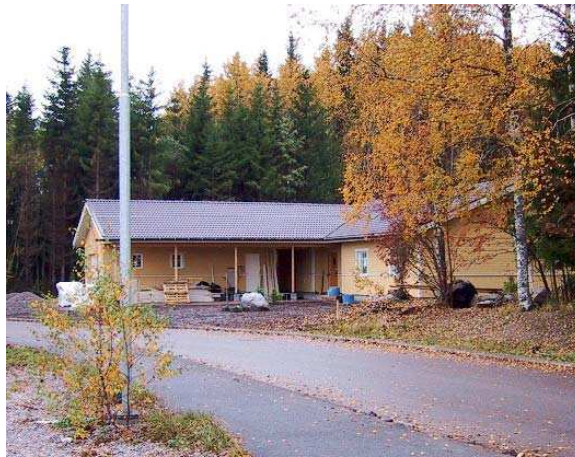
Figure 5. A building with completed exterior, and insulation waiting to be installed – example of continuous change causing nonconformity to completeness or temporal validity?
