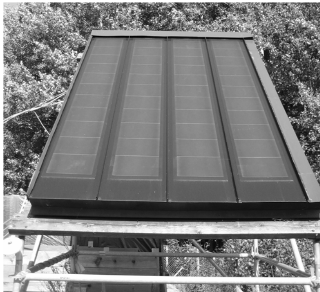
Figure 3. Four triple-junction a-Si modules installed on a free-standing metal roof tilted southwards at angle of 45°. The module type is Uni-Solar 64 W p PV-laminate with a butyl adhesive, and they are attached to a standard black painted metal roof manufactured by Ruukki.
