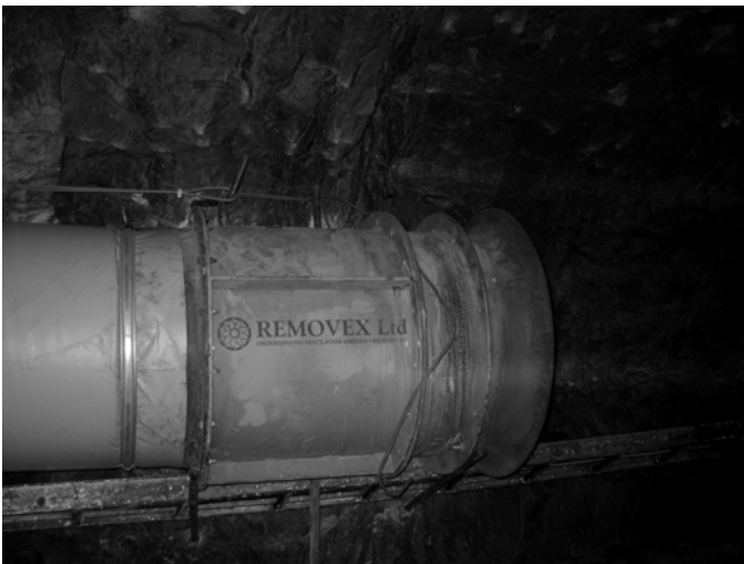
Figure 1. An additional fan installed on level +130 m.
