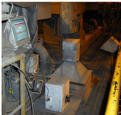
Fig. 2. The actual system running in Pyhäsalmi concentrator
