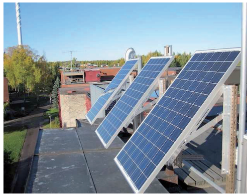
Figure 3 Main solar panels, 3 x Naps NR100G24.
